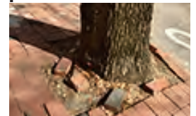
Tree pit too small for rain to water this tree.
