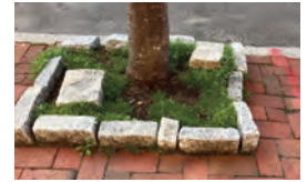
Belgian blocks around a tree pit present a tripping hazard.
